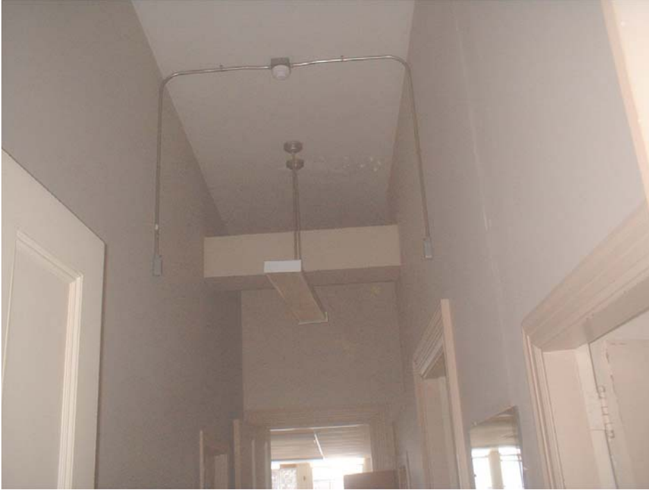
Interior, view of exposed wiring conduits.
