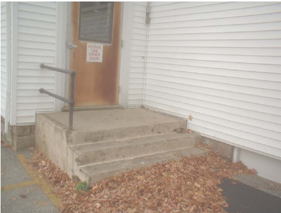
Exterior, detailed view of stairs. Non-accessible, no guardrails/handrails.
