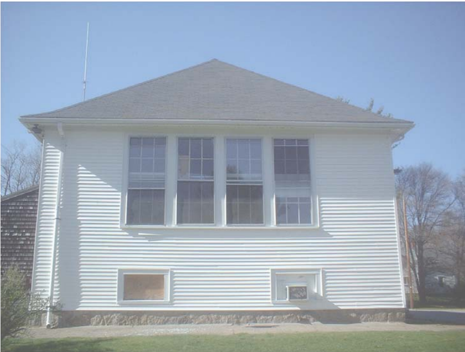
Exterior view of south facade, broken glass on ground.
