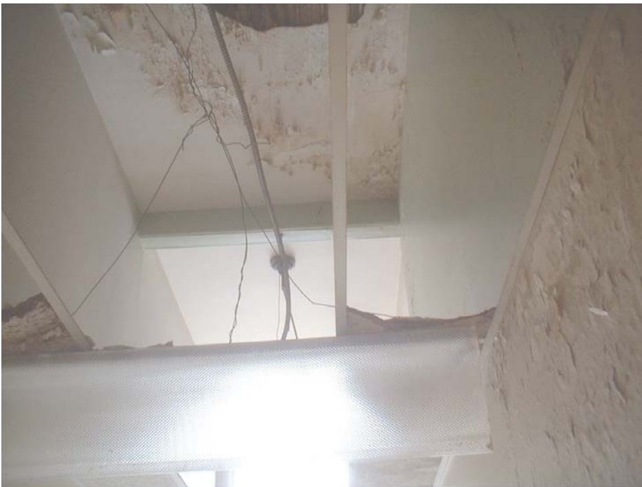
Interior, view of conditions of wall and ceiling in stairs.
